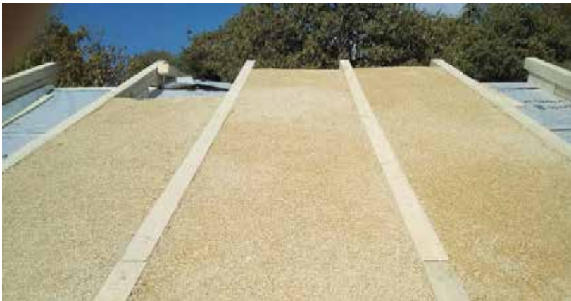
CANAPAMAS 385 Roof insulation
